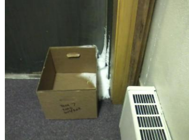
Snow blowing under fire escape door
